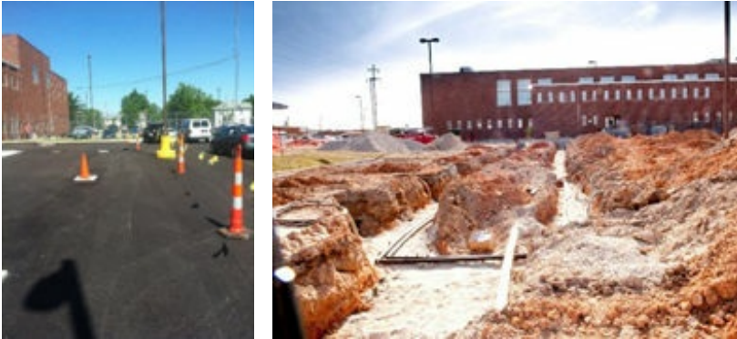
The existing parking lot served as the location of the geothermal system well field and a newly paved lot at the end of the project.
