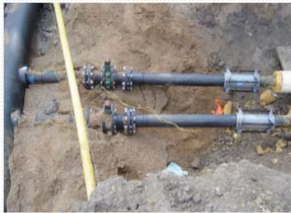
Well pipes in the first of three geothermal well fields – 140 wells, each reaching 350 feet deep – work to generate the first 240 tons of what will grow to generate 1,200 tons of cooling.
