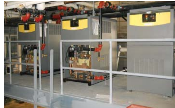
↑ New Condensing Hot Water Boilers
