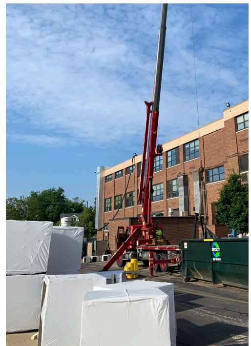
Preparing to lift new roof top HVAC units onto the roof at McHenry East High School.
