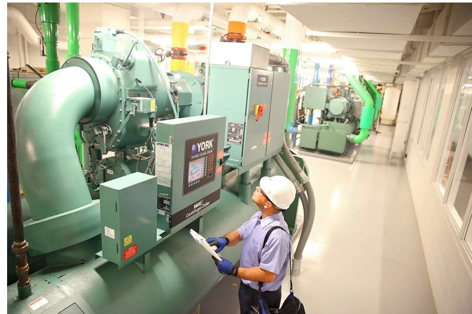
Johnson Controls, Inc. Chiller Improvement
